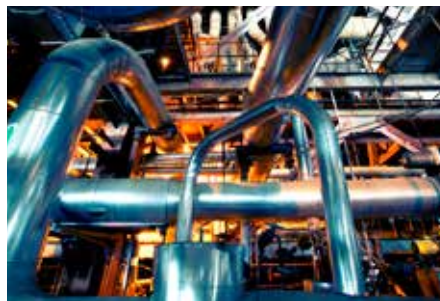
Power plant operations
